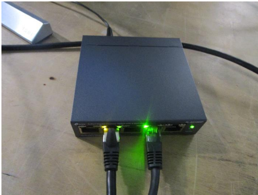
Photo 8: Support Equipment – Ethernet switch
